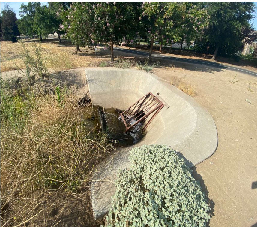
Photograph 4: Western end of ditch with concrete apron where water re-enters the subsurface pipe, looking southwest.
