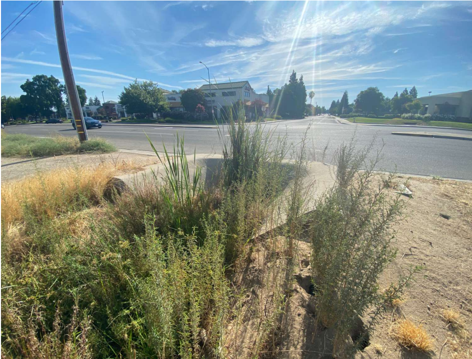
Photograph 1: Eastern end of ditch and concrete apron where the conveyance daylights. View east with N. Clovis Avenue (mid-ground) and Palo Alto Avenue (background) visible.
