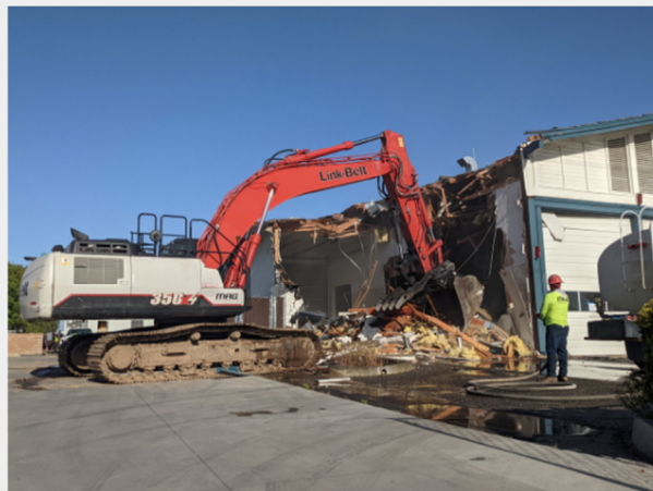
Demolition: Fire Staff assisted the construction crew to demo the nearly 50 year old station in April 2023.
